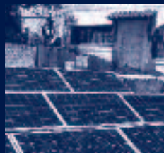
2.1 kWp PV plant fitted with ConSole
